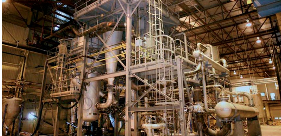
Pyrolytic liquid platform biorefinery for polymers, synthetic fuels, food, power and heat from lignocellulosic residues. Courtesy Ensyn, Canada; and Task 42.
