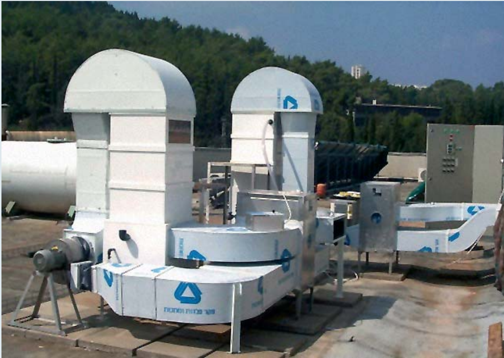
Figure 16: 20 kW liquid desiccant system, Energy Engineering Research Center Building, Haifa. (source: G. Grossman, Technion Haifa/Israel)
