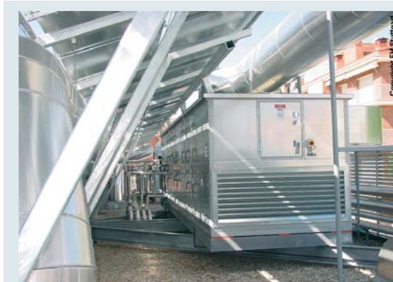
Figure 13: DCS unit mounted on the roof at Mataró Library (source: FH Stuttgart)
