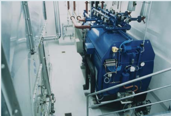
Figure 9: Adsorption chiller at the University Hospital of Freiburg (source: Fraunhofer ISE/Freiburg)
