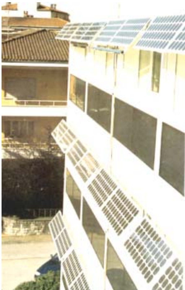
Figure 2: PV modules mounted on a facade as shading elements and for electricity generation
