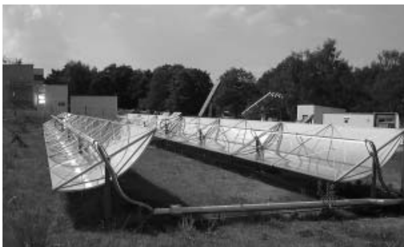
Figure 12: IST-Trough collector at DLR, Cologne
