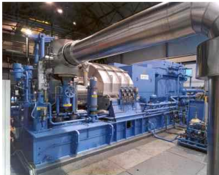
Figure 7: A condensation steam turbine with 10 MW el
