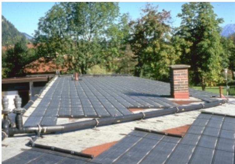
Figure 4: Plastic absorber for swimming pool heating
